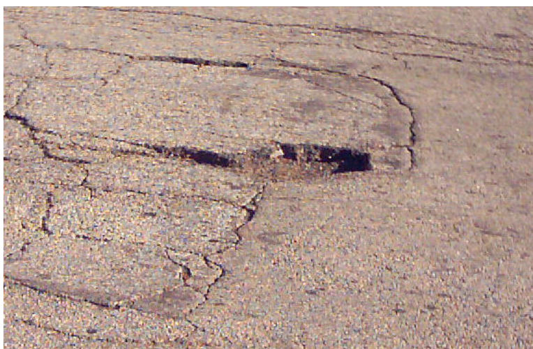
Figure 9.1: You can see the once smooth road surface has cracks and fractures, plus a large pothole. (11)
